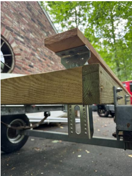
Figure 4: Installing bunk brackets on the existing wooden frame. Carpet was added to the bunks later.
